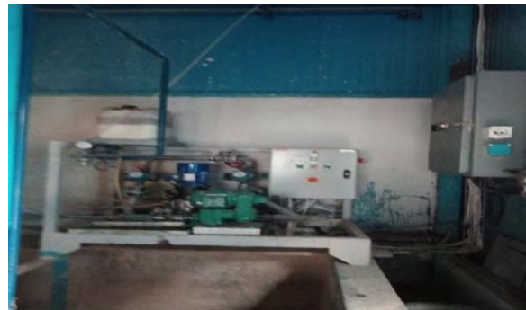
(b) Installation for polymer preparation
