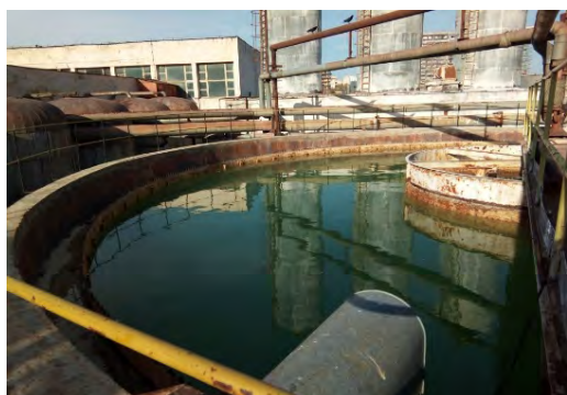
(a) View with lime tins, mechanical filters and primary radial settling tank
