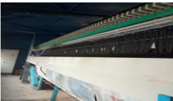
(c) Conveyor belt for sludge dehydration
