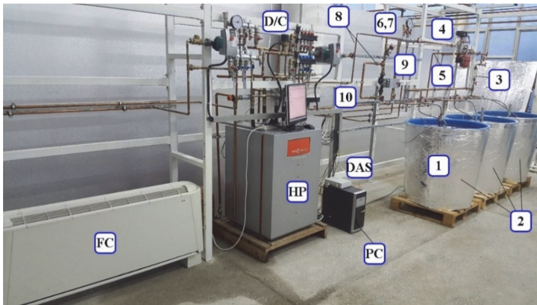
Fig. 8. The experimental stand - storage tanks and secondary circuit
