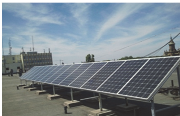
Fig. 4. Panels of the PV system
