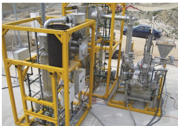
Fig. 2. General view of the gasification / vitrification unit
